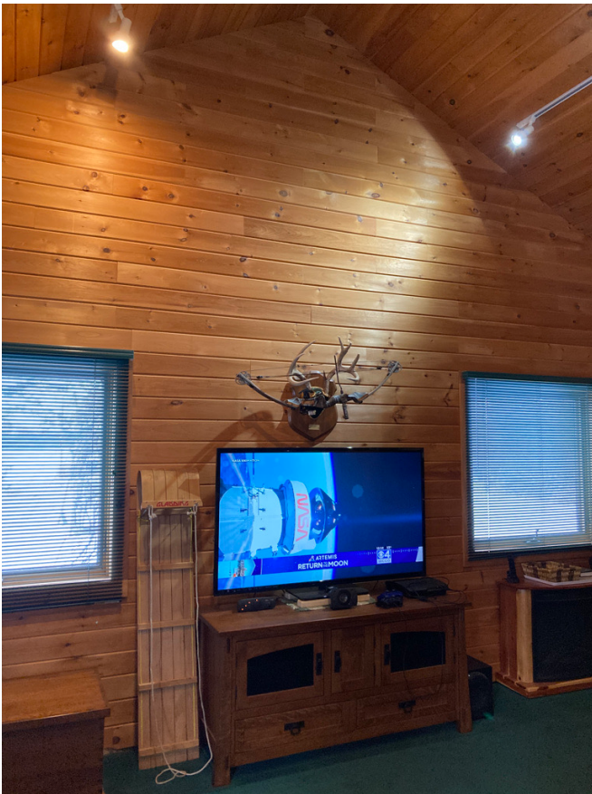
Interior finish of existing building. The intent is to preserve the naturally oxidized white pine interior. The interior height is 9' at sidewalls and 15' at center.
